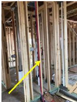
Missing PEX pipe insulation
