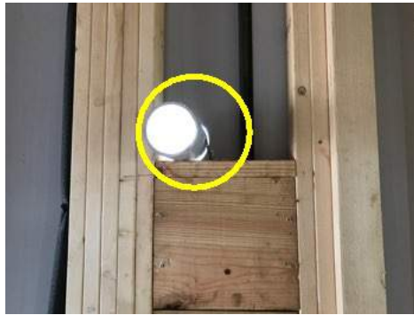
Seal around wall penetration
