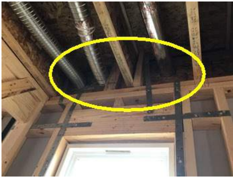
Seal around wall penetration
