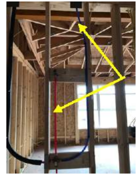
Missing PEX pipe insulation
