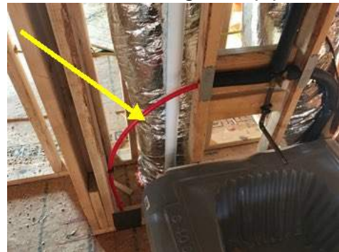
Missing PEX pipe insulation
