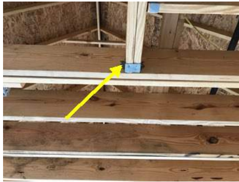
Missing nail floor joist support (garage)
