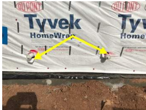
Tape around pipe penetration
