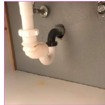
Accordion pipe (hallway bathroom)
