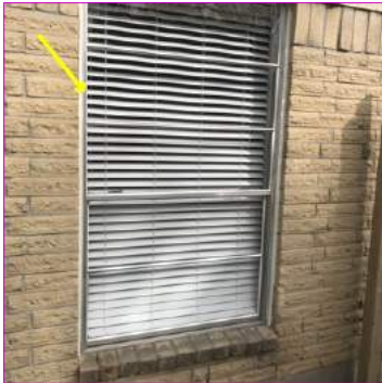
Seal gaps in window trim (left side)
