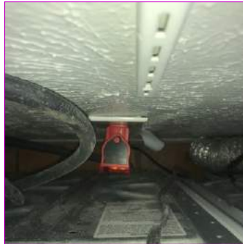
Receptacle not GFCI (laundry)
