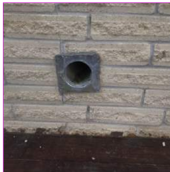
Dryer vent missing screen
