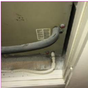
Missing secondary condensate drain
