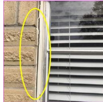
Seal gaps in window trim (zoomed)
