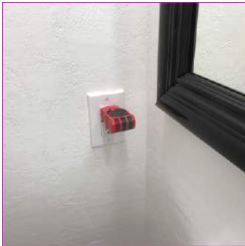
Inoperative GFCI receptacle (half bathroom)
