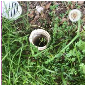
Broken clean out cover (back side)
