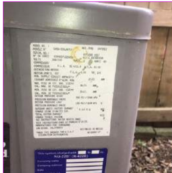
3 tons AC condenser S/N
