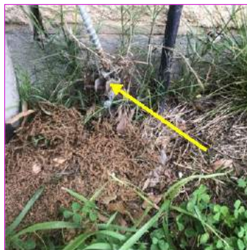
Service grounding ok
