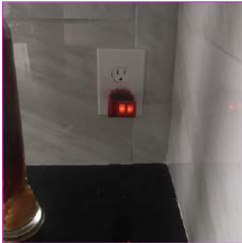
Receptacle not GFCI (kitchen)
