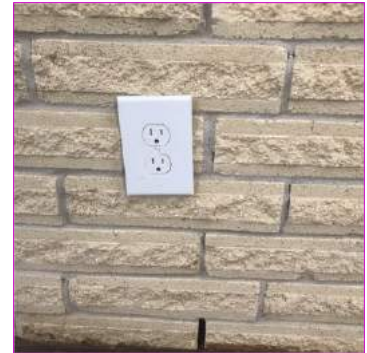
Exterior receptacle not GFCI (back side)
