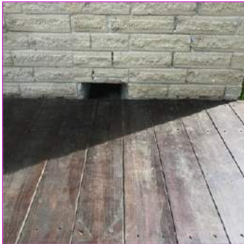
Missing ash clean out door (Chimney)
