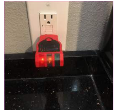
GFCI hot/neutral reversed (hallway bathroom)
