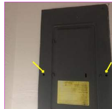
Missing front cover screws
