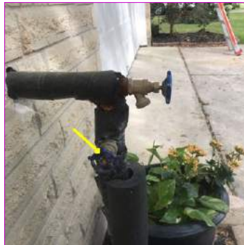
Main water shut off valve
