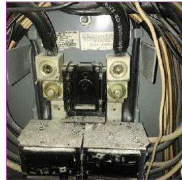
Aluminum service wires missing anti oxidant
